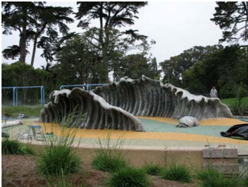
Wave walls by Peterson Architectural Arts are ready for final finishing coat. (View east)
