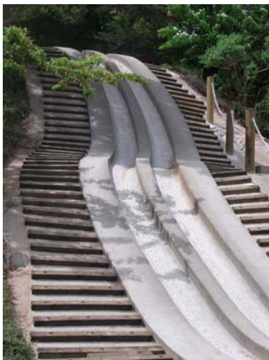
Hillside slides have been renovated with new steps and rails. (View south)
